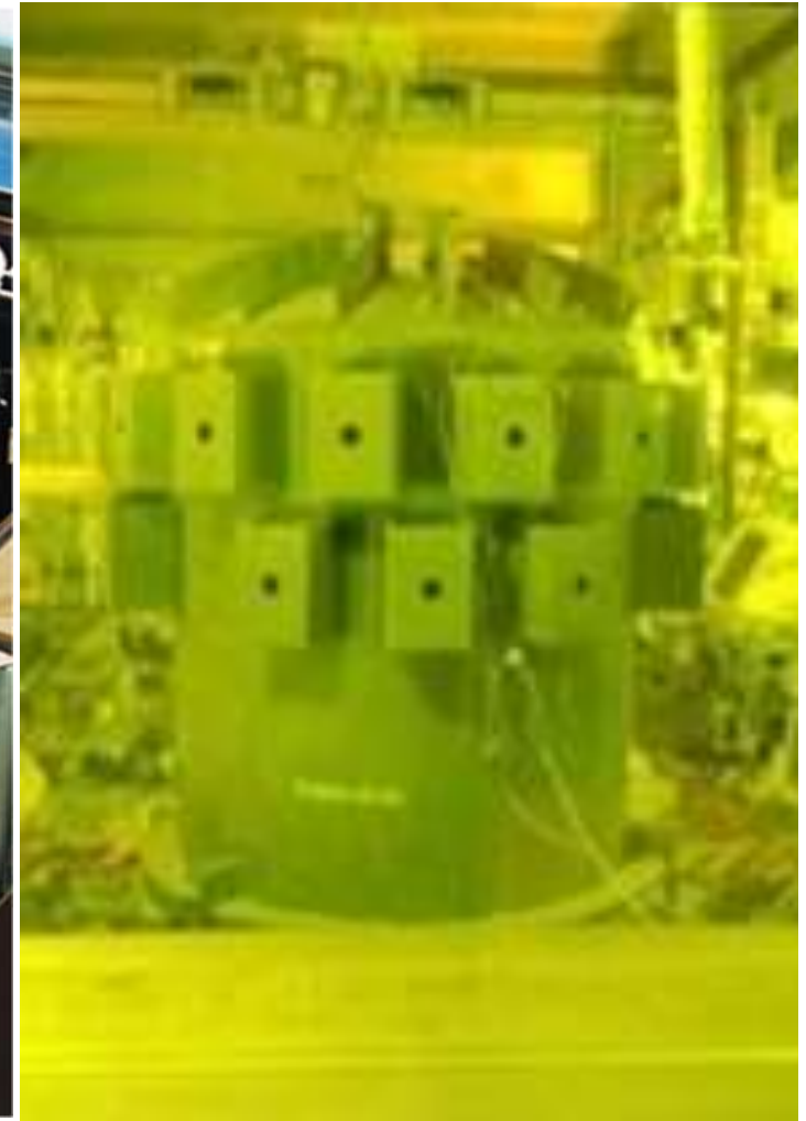
Metal Waste Furnace
